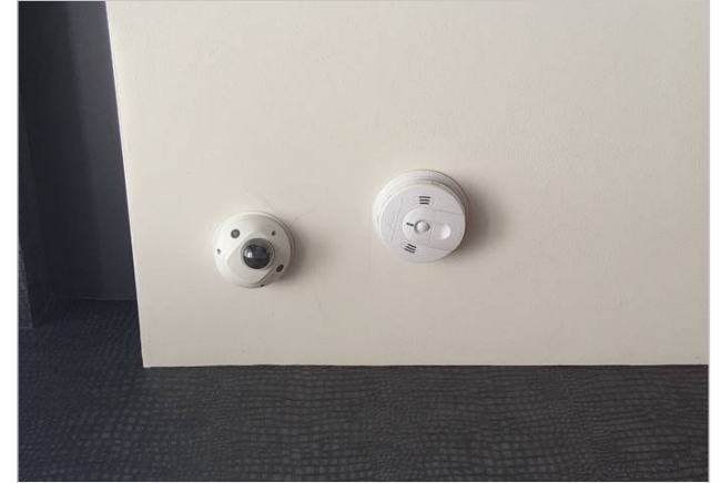
Fire Protection/Alarm systems 10.3
